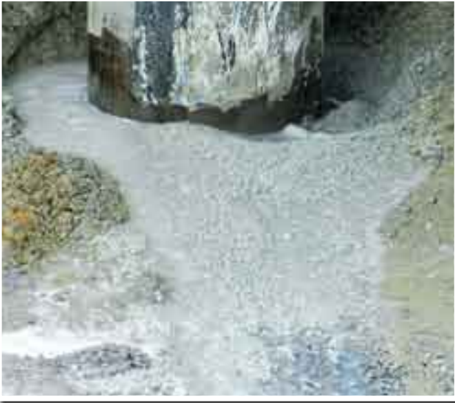
The EZ-SEAL® bentonite grout slurry has been pumped down 17 feet through a tremie pipe into the bottom of the annular space around the 16-inch casing and is shown flowing out onto the ground surface indicating that the annular space is completely full of grout.
