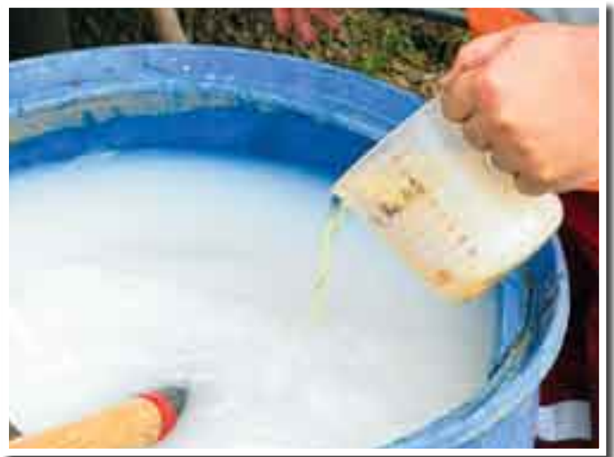
Adding the AQF-2™ foaming agent to 50 gallons of a water and QUIK MUD® D-50 polymer mixture that has an increased viscosity. This 3-component liquid mixture was injected into the compressed air stream to create the "stiff foam".
