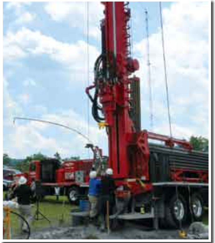
Installing the white 1-inch diameter PVC plastic tremie pipe to the bottom of the annular space between the 6-inch casing and the 10-inch borehole. A hose will connect the tremie pipe to the pump on the grout mixing unit.
