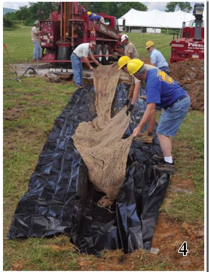
4. Placing jute erosion matting in the bottom of the plastic-lined trench. The fibers in the woven strands of the jute mat provide ideal attachment locations for the treated sediment flocs to grab onto as they flow by in the water.
