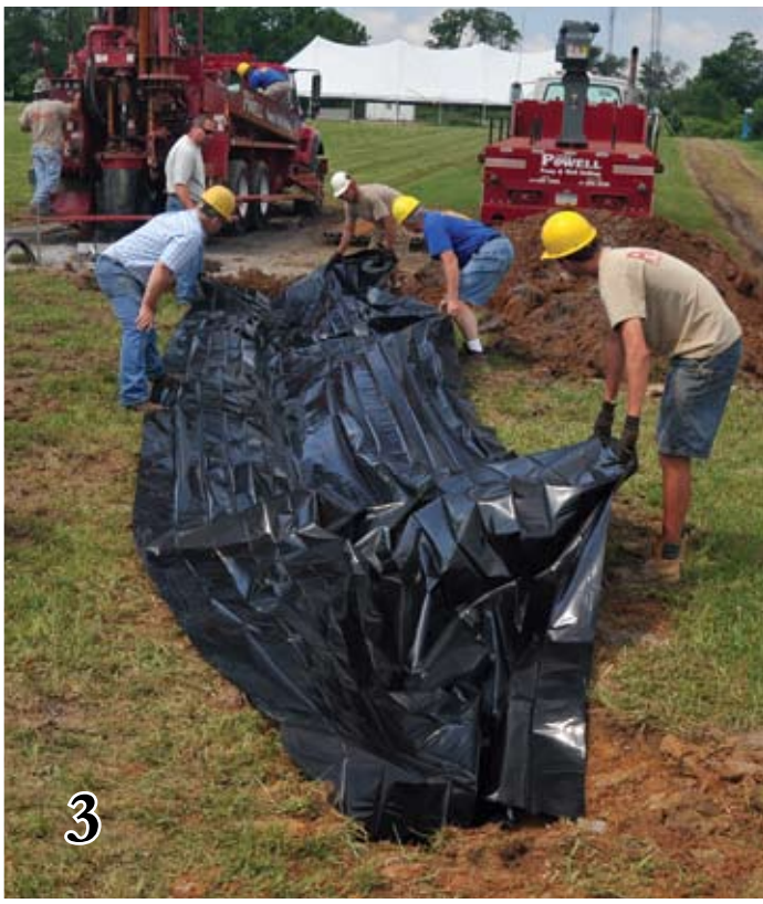
3. Lining the treatment trench with a heavy plastic sheet. Bentonite clay was used at the settling pit to seal the plastic sheet to the soil.
